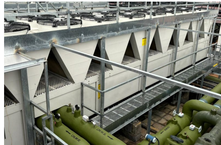
Replacement of variable speed drive chiller units at Tsuen Wan Government Offices
