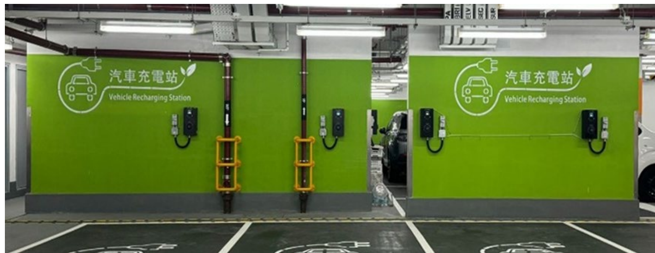
EV chargers at Treasury Building car park
