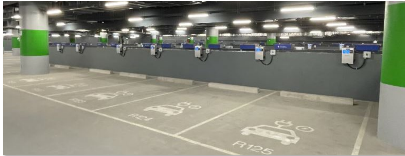
EV chargers at HYW BCP public car park
