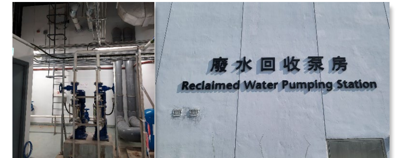
Rainwater harvesting system and reclaimed water pumping station at HZMB HKP
