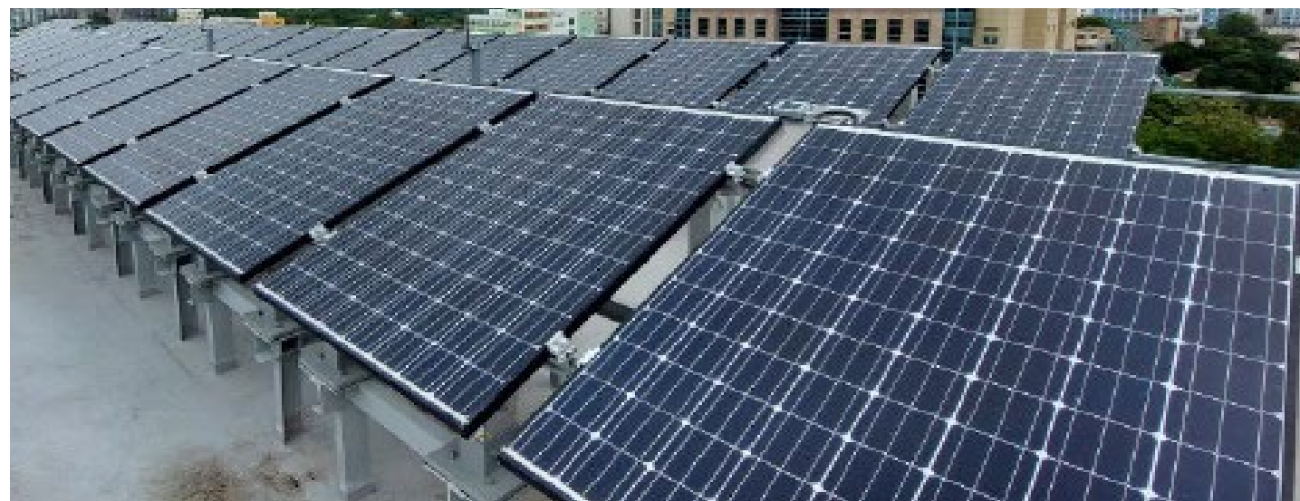
Photovoltaic panel system at North District Government Offices
