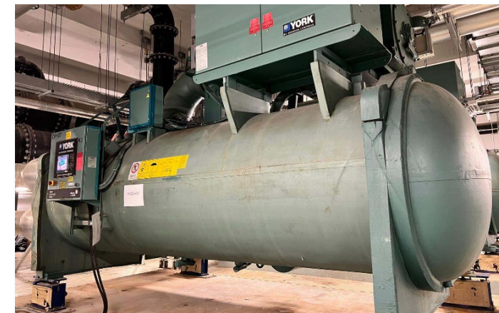
Seawater-cooled chillers at HZMB HKP
