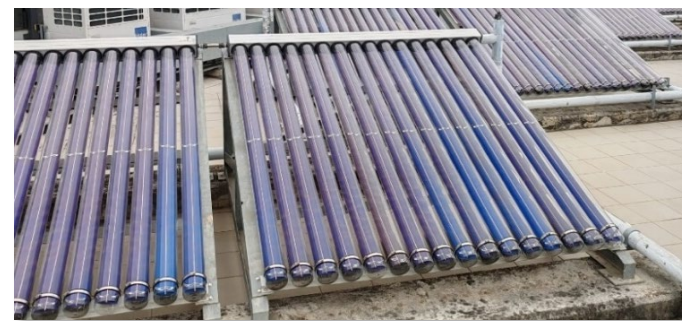
Solar hot water heating system at Heung Yuen Wai Boundary Control Point (HYW BCP)
