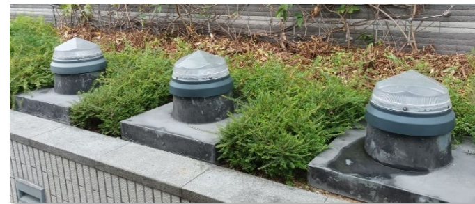
Light pipes at West Kowloon Government Offices
